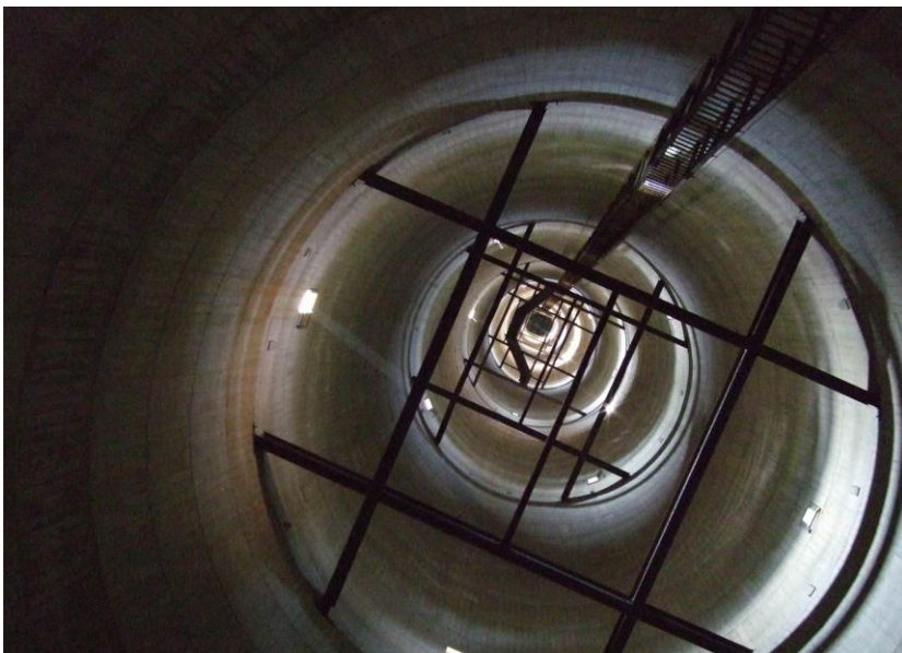
Fig.4 Inside of wireless tower
