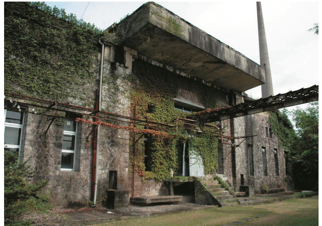
Fig.5 The current transmission room
